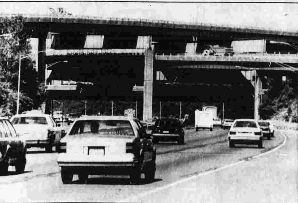
"STACKS" — This 20-year-old, three-level bridge over Interstate 84 that has never been used may cost state taxpayers $5 million to rehabilitate. Story on page 8.
